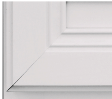
separation of door corner
