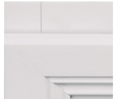
separation of frame joint
